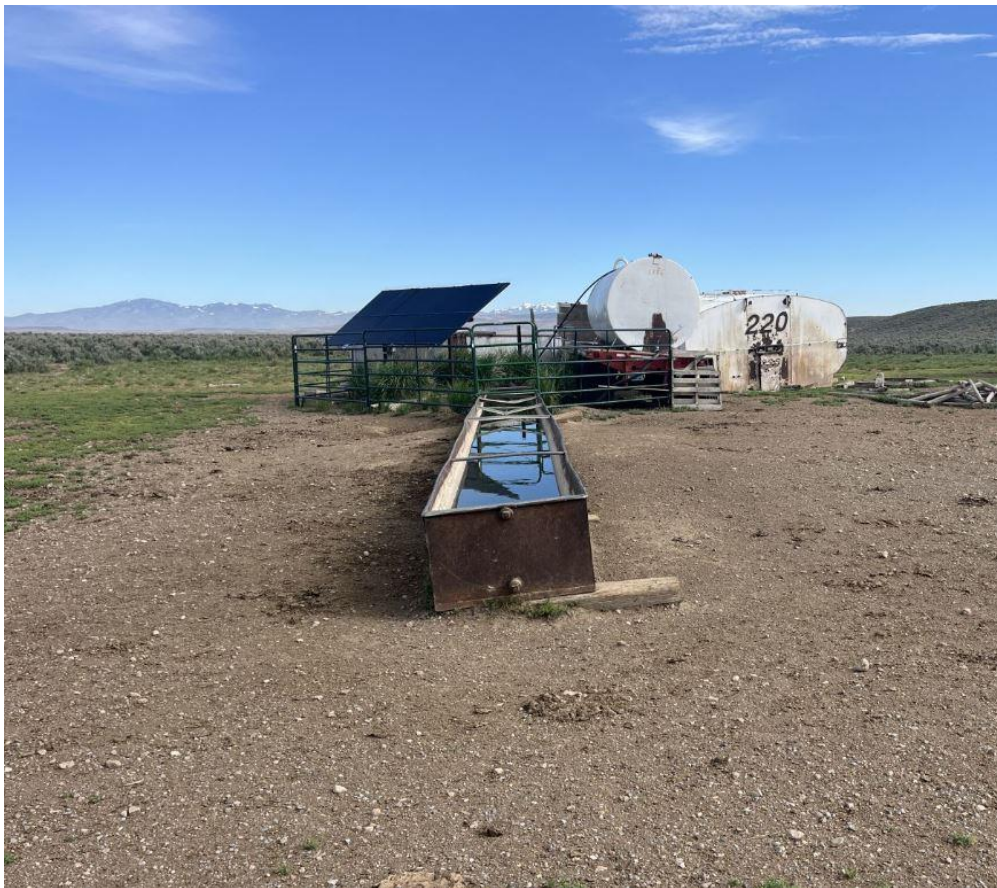
One of the stock wells powered with solar panels and pump with water storage tanks.
